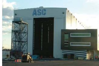
Work on our new facility at Henderson, Western Australia is nearly complete.
